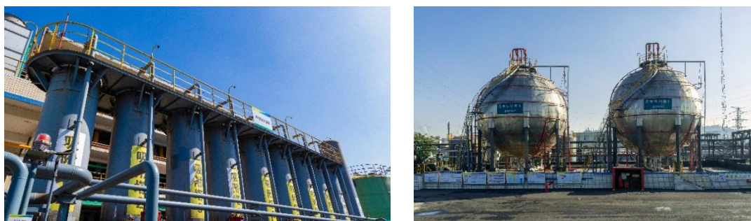
Figure 3. Chloromethane pressure swing adsorption unit and ball tank
