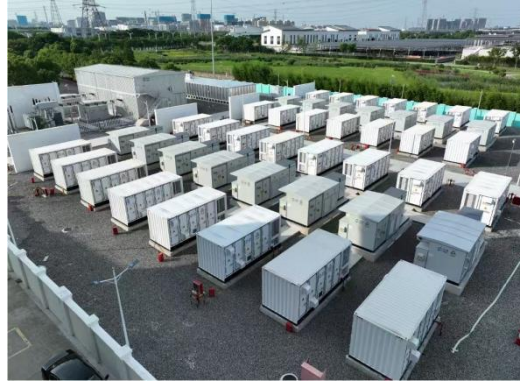
Figure 1 50 MW/100 MWh grid-side energy storage project of Suzhou Shengneng
